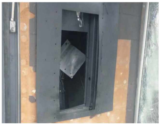
A hole in the wall where the ATM sat before it was blasted apart in Nigel Road, Selcourt on Saturday.
